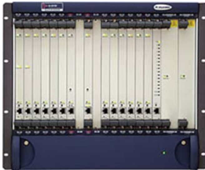
Figura 10 Soft Switch Softx3000 Huawei.
