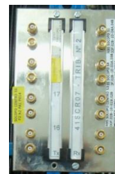
Figura 31. Panel de conectores E1's Rack DDF.
