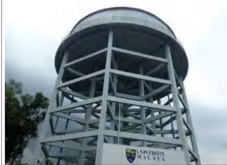
Tangki Simpanan Menara Utama (Apartment Jepun) Capacity: 2,000 m 3
